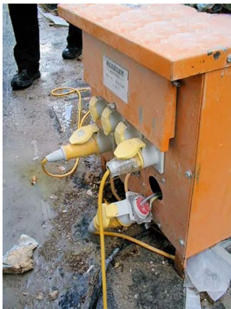
Broken plug on transformer.
