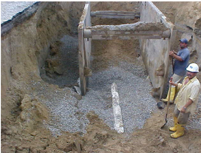
Trench Box - Wonder why these contractors are not on approved list anymore?
