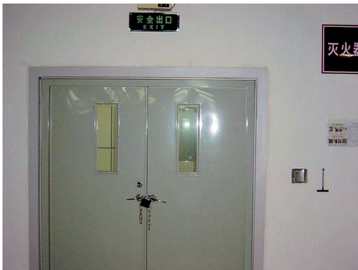
Locked fire exit
