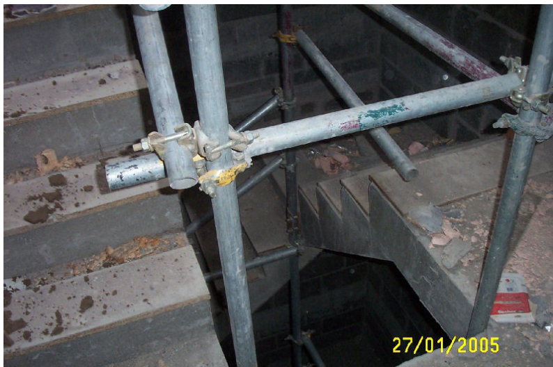
No edge protection, handrails and a few trip hazards! More...
