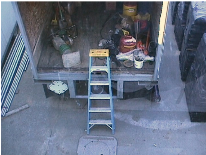
Transport safety - Incorrect use of step ladder.
